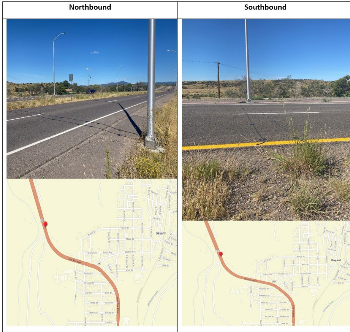
Figure 27. JAMAR Counter, North of Bayard (Esri, HERE, Garmin, FAO, NOAA, USGS, OpenStreetMap contributors, and the GIS User Community, 2023)
